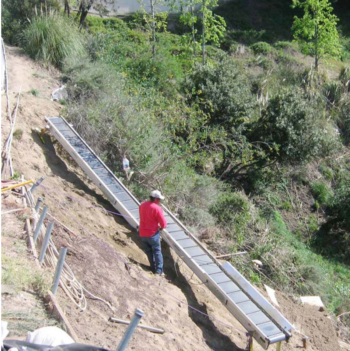
FIGURE 8 Example of Portable Conveyor System for Moving Sand up an Incline.
