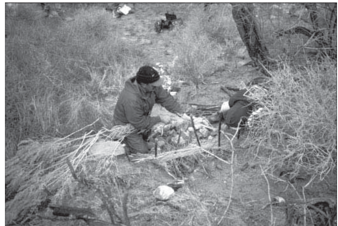
Figure 6. Members of the Zuni Soil Conservation Project constructing a check dam by using the basket-weave technique (photograph courtesy of Grand Canyon National Park).
