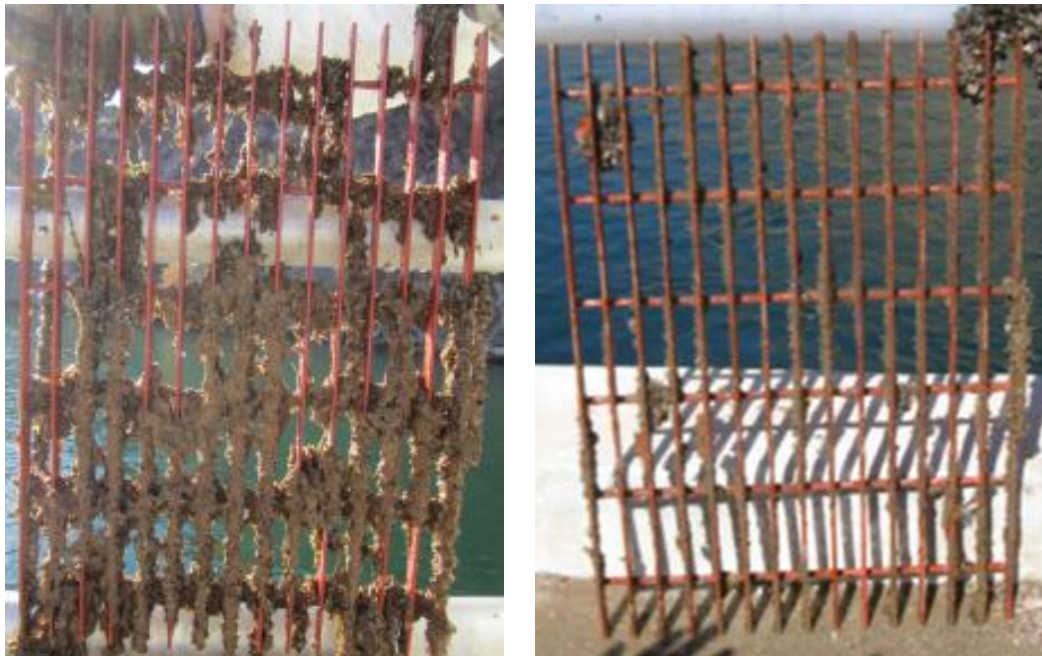
Figure 8. Grate coated with Silicone Epoxy #7, as seen in December 2013 (left) and in May 2014, after 1 year of exposure (right).
