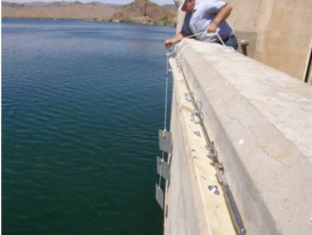
Figure 2. Coated steel plates placed in static exposure from the face of Parker Dam.
